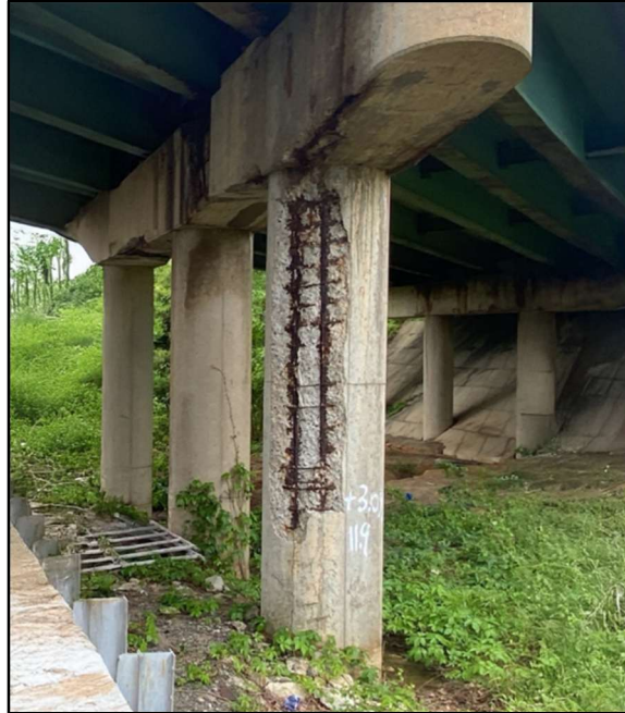
Figure 2: Existing Bridge with Corrosion (Source: ASCE)
