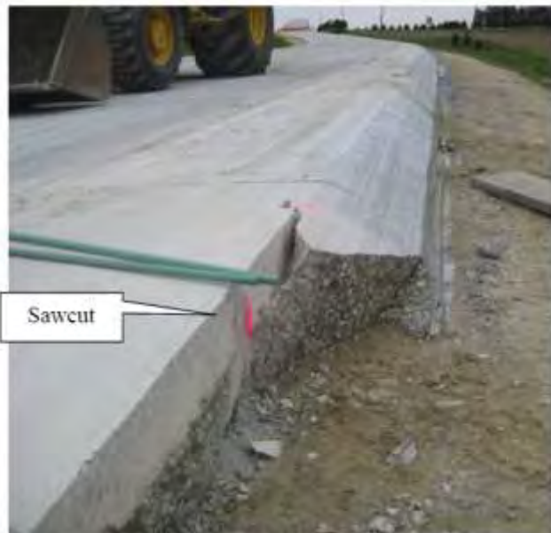
Figure 4. Sawcut on a PCC project at an intersection to remove the Safety Edge SM .
