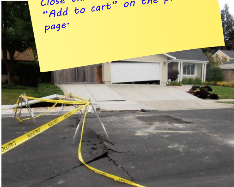
Figure 2-5 A dwelling damaged due to fault movement in the 2014 South Napa Earthquake. (from Geotechnical Extreme Events Reconnaissance, GEER)
