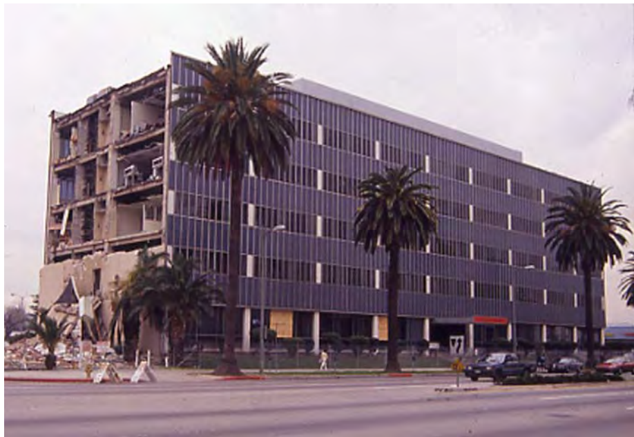
Figure 6-3 Partially collapsed end-wall in 5-story office building caused by severe earthquake ground shaking. (C. Arnold photo)
