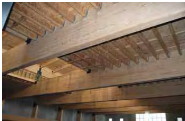
Figure 1. Wood-based composites used in the new Centennial Research Facility at the Forest Products Laboratory. Glulam timbers support composite I-joists and plywood sheathing. (Photo by Steve Schmieding, Forest Products Laboratory.)
