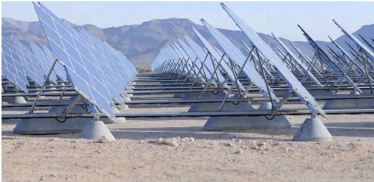
Figure 3. Single axis sun-tracking mounting structure, concrete footings, support beams, and PV panels at Nellis Air Force Base, NV
