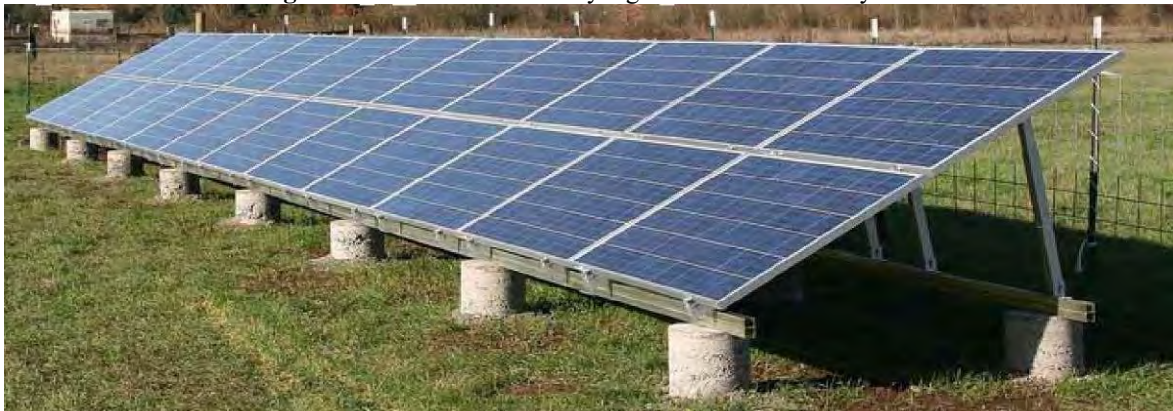
Figure 1. Fixed tilt A-frame style ground mounted PV system
