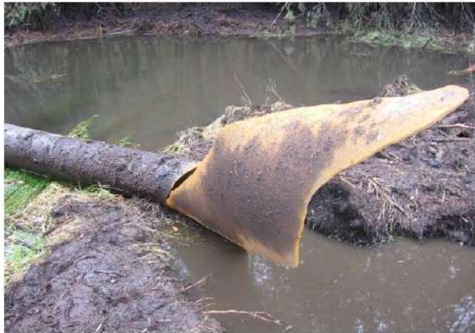
Figure 5: End of severed 37.1 foot section of pipeline
