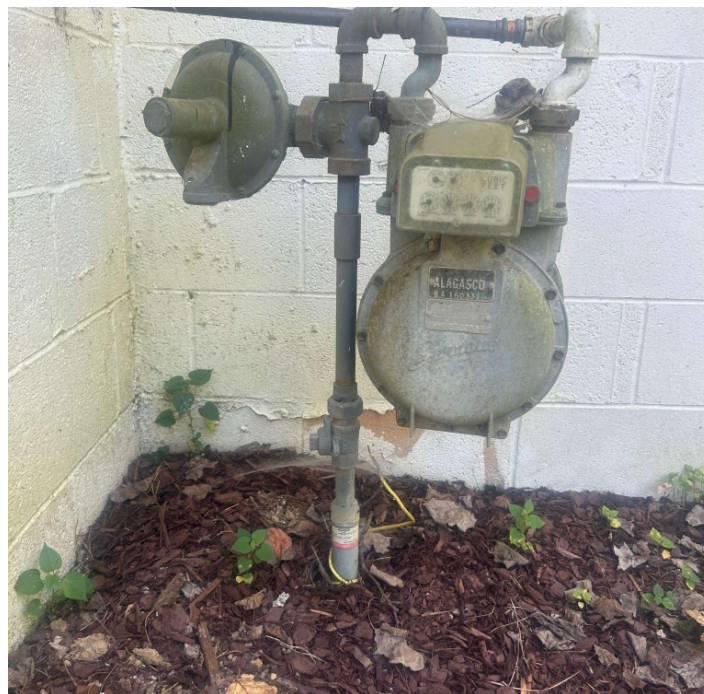
Figure 3 - A common diaphragm meter found at just about every residential property. Source: Robert Noriega (self)
