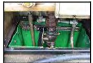
Contained dispenser sump
