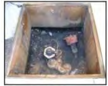
Uncontained turbine sump
