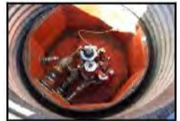
Contained turbine sump
