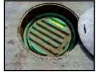
Circular steel sump lid pulled back to show the inner lid covering the turbine sump
