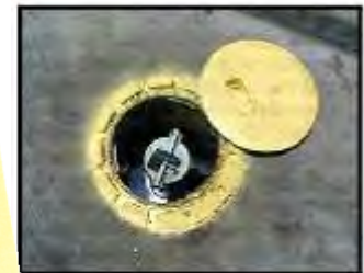
Circular spill bucket lid pulled back to show the fill port with a spill bucket
