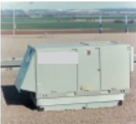
Figure 11: Small rooftop air handling unit.
