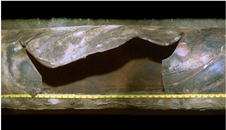
Figure 1: Bellingham Rupture Site
