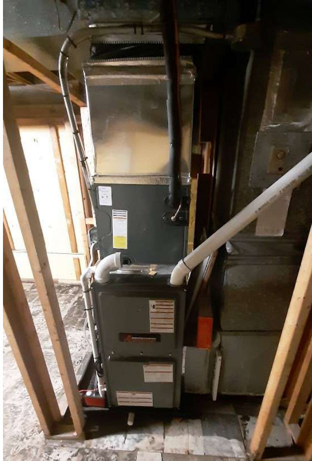
Power Vent Gas Furnace
