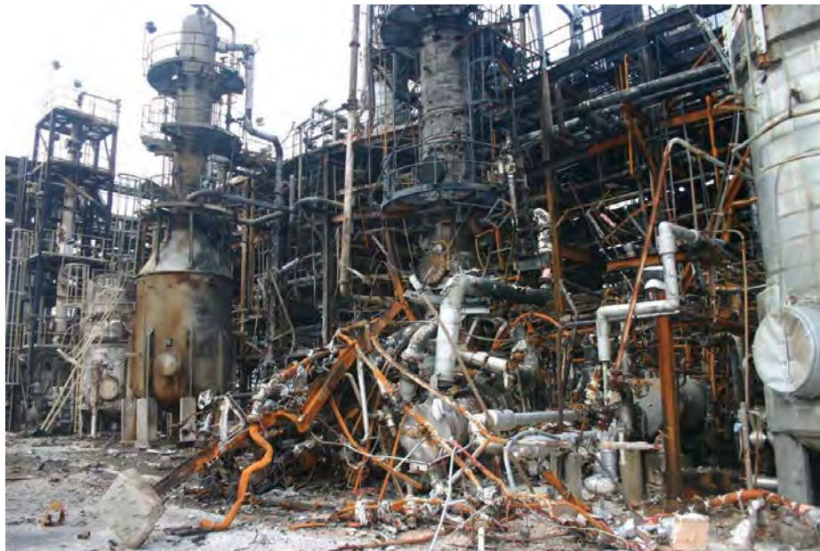
The explosion ripped out piping, electrical conduit and damaged structures in the facility. (Source: CSB Report.)
