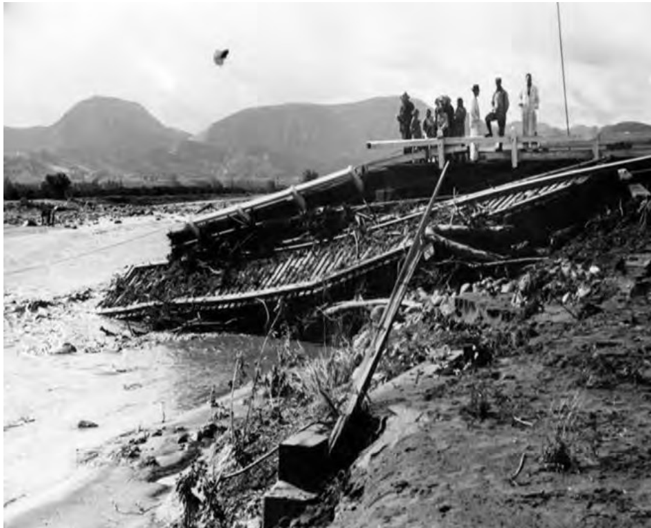
People examine the damaged road and washed away railroad track, caused by excess water flowing down the Santa Clara River after the failure of the St. Francis Dam.
