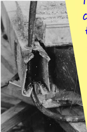
Figure 3 - Fourth Floor Box Beam Connection. The rod slipped through the box beam, resulting in the collapse of the walkway (see Figure 3).
