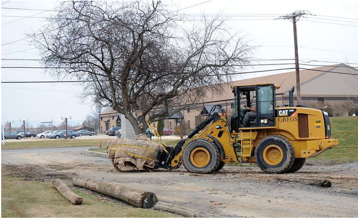
Figure 1: Front loader relocating a large tree and root ball as part of a construction project, in accordance with an environmental permit.
