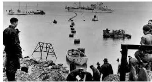
Photo of Gotland Sweden HVDC link in 1954.
