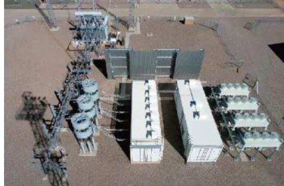
Photo of an Operating STATCOM System
