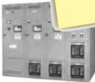
Figure 4: Service entrance with transfer switch (floor-mounted).
