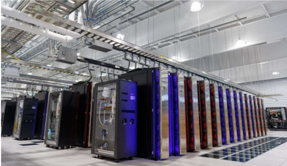
Figure 3: Rack Layout (Source: DOE – Federal Energy Management Program)
