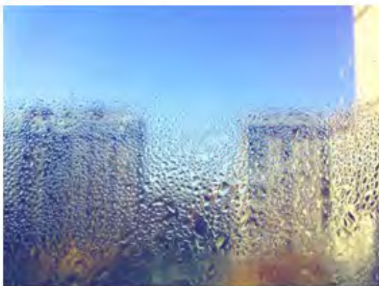
Window Condensation with High Indoor Humidity
