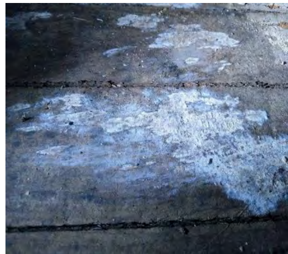
Mold Heralding a Moisture Problem
