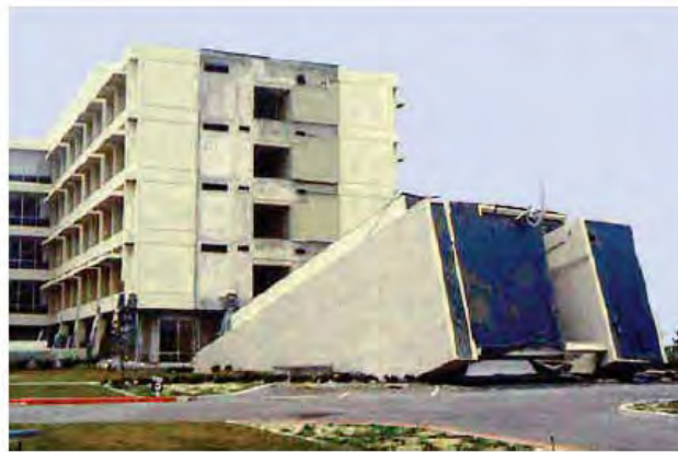
Figure 2: Olive View Hospital. A brand new facility that was damaged beyond repair in the 1971 San Fernando earthquake due to a shaking intensity that exceeded what was expected at the site and a design that, although technically complying with code at the time, contained several structural characteristics now considered major deficiencies. The lateral system contained nonductile concrete frames, discontinuous shear walls, and a significant weak story.
