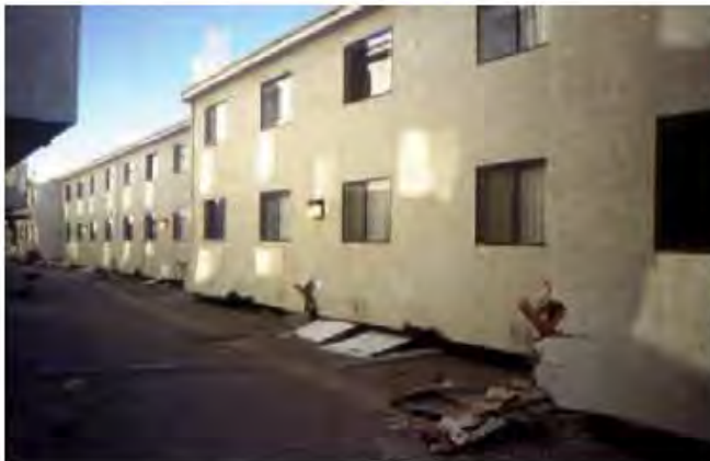
Figure 5: A tuck-under similar to Figure 8-4, but much more modern and designed at a time when the weakness of the parking level was more understood. In this case, the detailing of the small wood shear walls at that level was poor. This practice created another set of deficient “existing” buildings.
