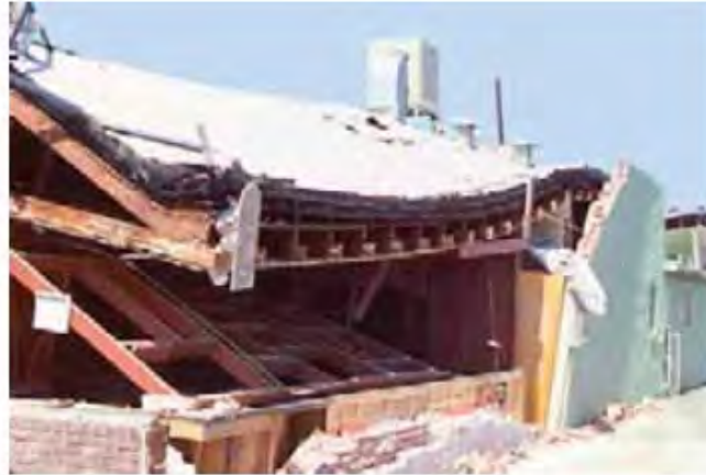
Figure 1: Example of buildings with no code design. Damage shows classic URM deficiencies.
