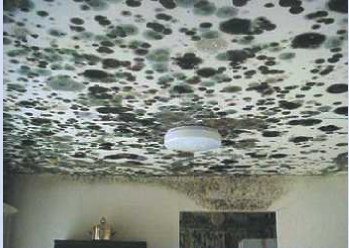
Photo 1: Extensive mold contamination of ceiling and walls
