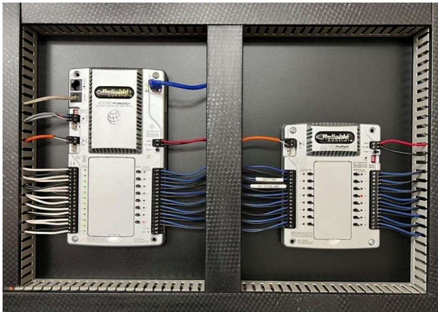
Figure 2: Direct Digital Control (DDC) System Panel
