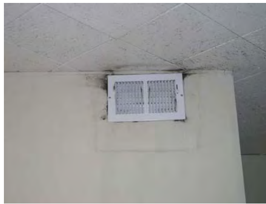
Figure No. 5 – Mold at Supply Grille
