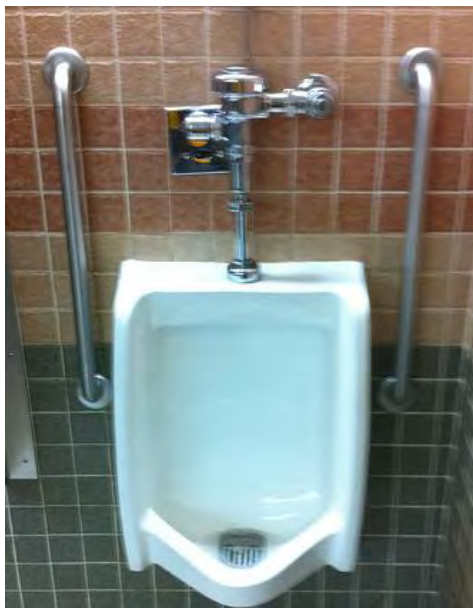
Figure 4 – Toilet rooms with one urinal will no longer be required to provide an accessible urinal.
