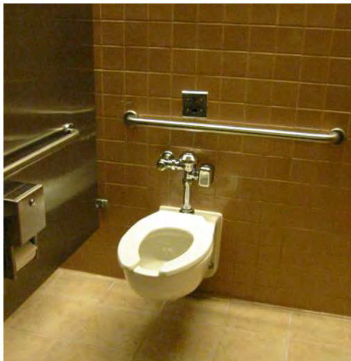
Figure 2 – The DOJ is considering the need for multiple wheelchair accessible compartments in toilet rooms serving airports and train stations because of travelers with luggage.
